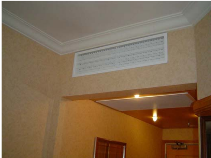
Figure 3. Photograph of installation of the active chilled beam in the test room
