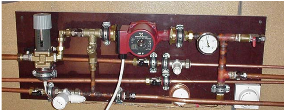
Figure 2. Photograph of the mixing system
